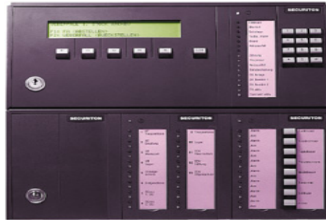
Fire Alarm Panel
